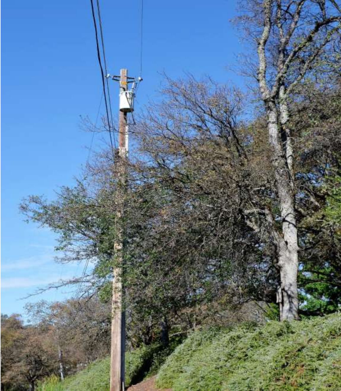
Heavy vegetation surrounding powerlines.
